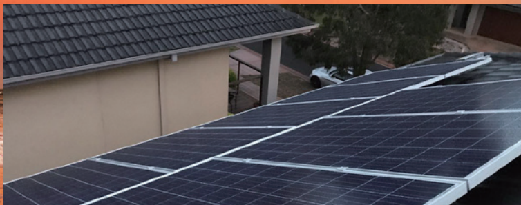
3.6KW | Melbourne, Australia
